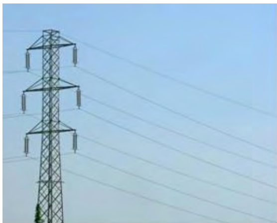
Fig. 6: Tralicci AT piramidali.
