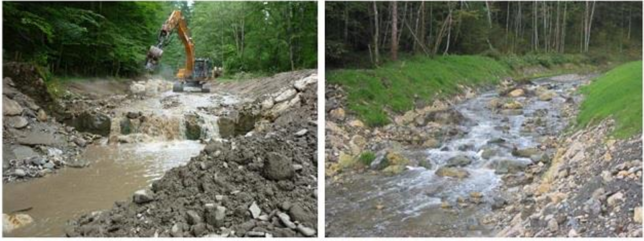
Illustration22 - During and after the reconstruction (ramp with height 1,6 m and length 70 m).
