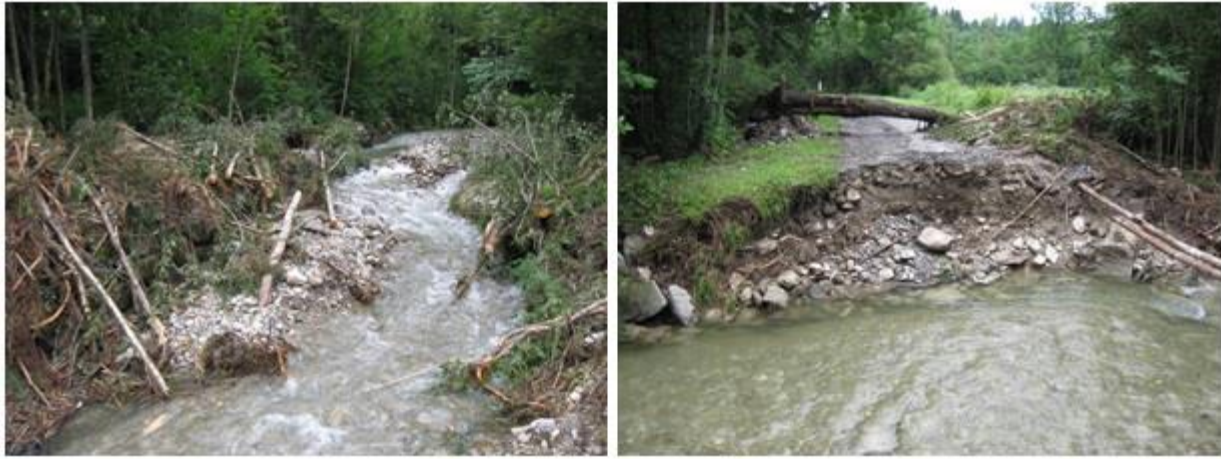
Illustration20 - Wood log jam destroyed a bridge; also several check dams are damaged
