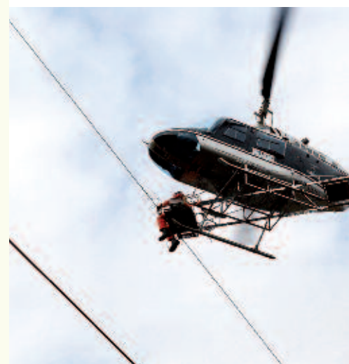
Implementation of colored spirals on a high voltage "Stagni della Piana Fiorentina e Pratese" and in part (Campi Bisenzio-Fi) to mitigate the impact on birds. The operation was made possible thanks to an agreement...
