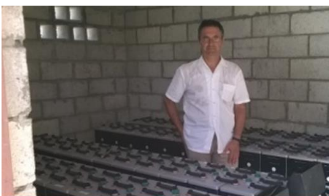
ENEA technician visiting the solar installation financed by IMELS at the Chevalier College. Kiribati, March 2017
