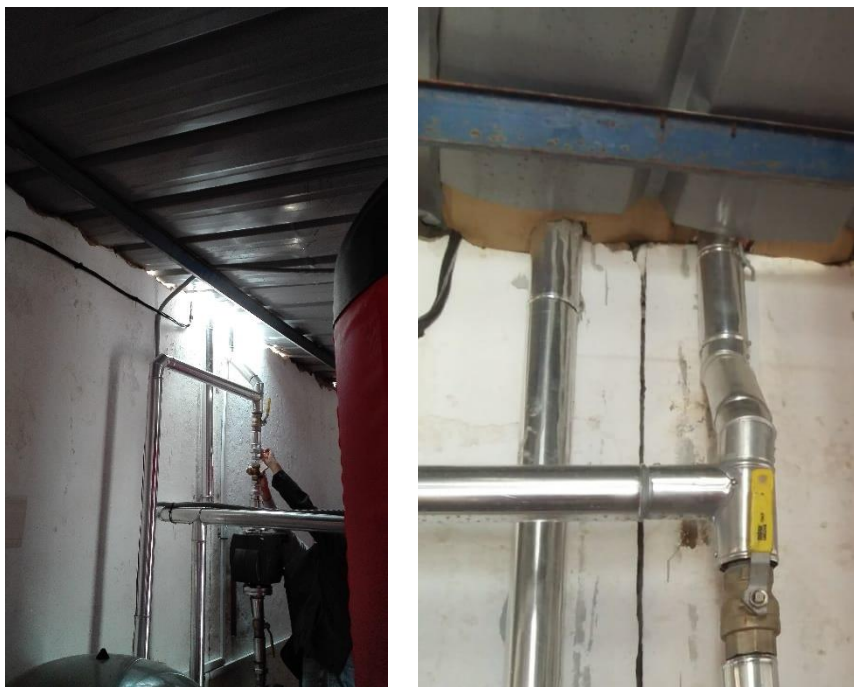
Figure 2.5: Cuisine Centrale technical room.
