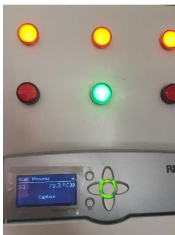
Figure 3.10: Internat Faidouzi electrical panel.
