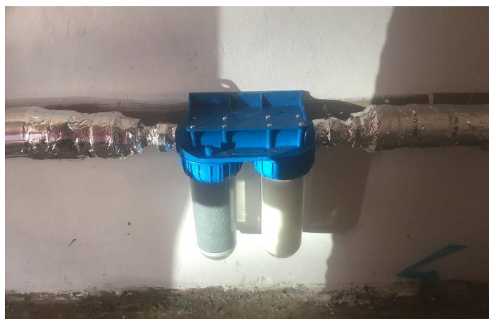
Figure 2.7: Cuisine Centrale additional filters.
