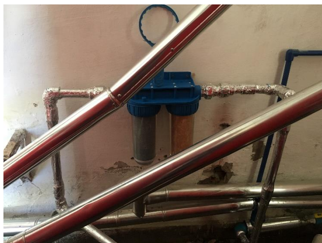
Figure 3.5: Internat Faidouzi additional filters.
