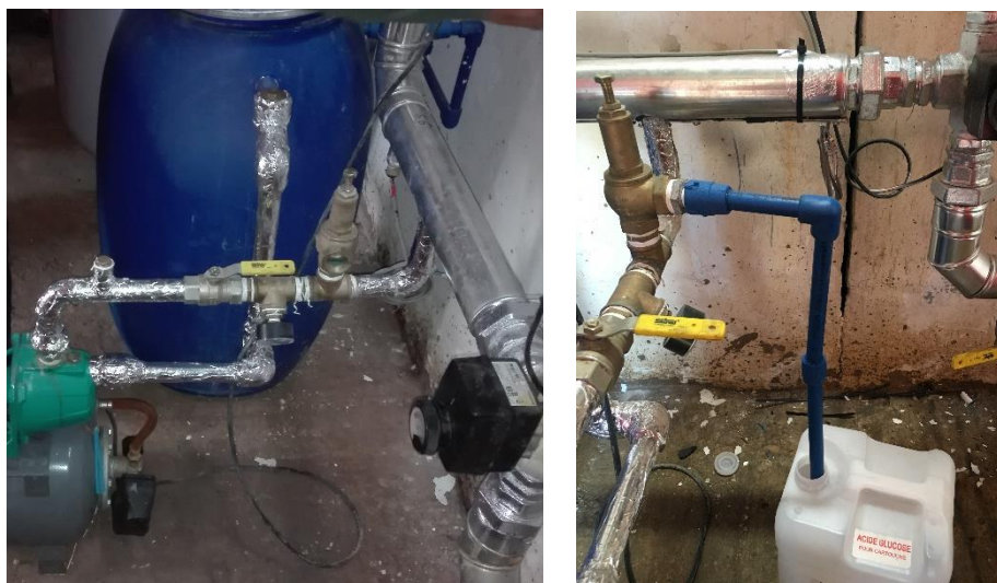
Figure 2.8: Cuisine Centrale collection system for solar safety valve..
