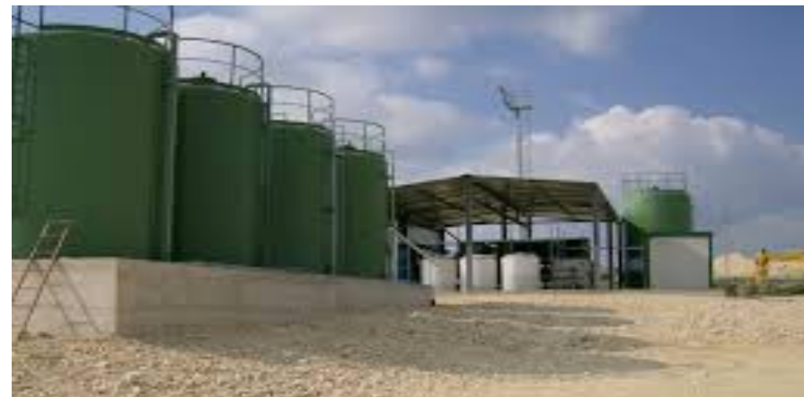
Leachate Treatment Unit
