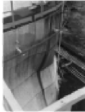
Damage to the wall of the gasoline tank
