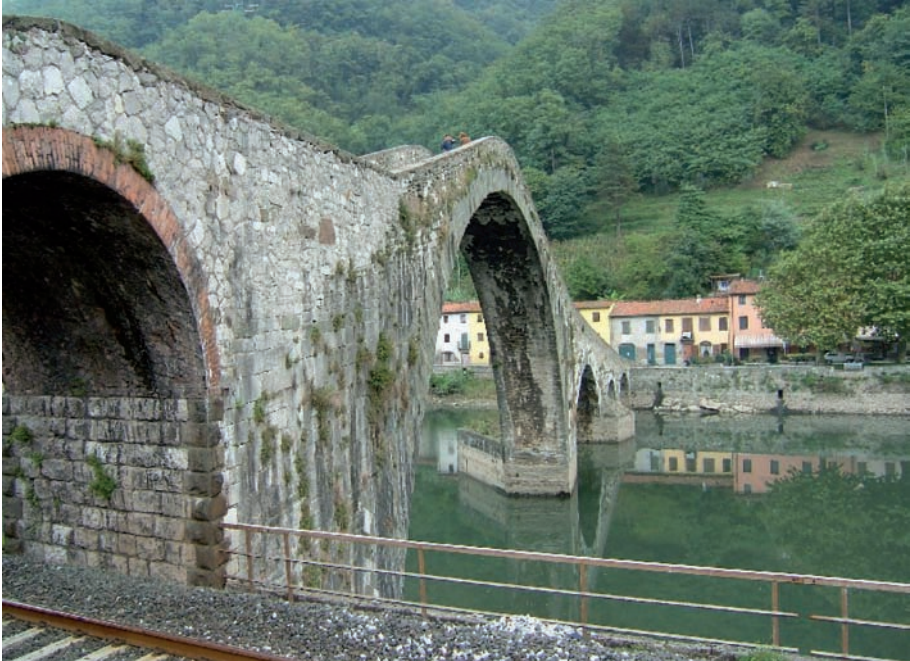
Figure 2.9 – Stone bridges such as this one often have spaces between stones suitable for roosting bats (Photo by P. Agnelli).
